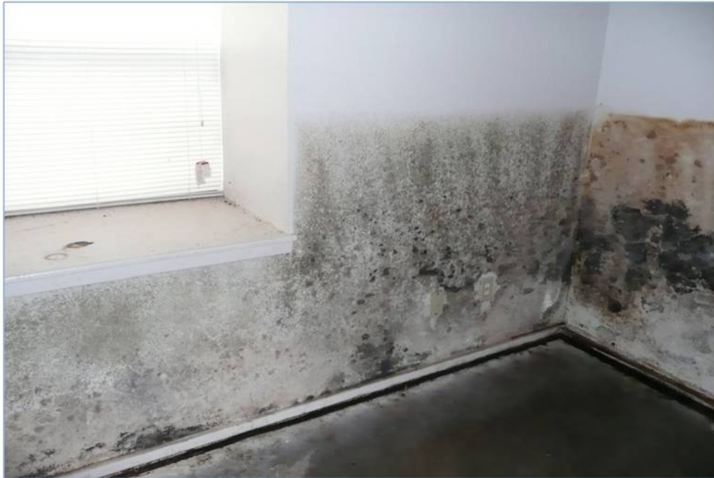
Figure. Interior Condition at Kristie Manor Apartments at time of Demolition Order and Substantial Damage Declaration. The buildings had flooded multiple times, each time experiencing further deterioration. Note the high water mark and mold. Had the apartment buildings been repaired without bringing it into compliance with the flood requirements, the structures and occupants would have remained at risk for this sort of damaging and life-threatening flooding due to their location in a floodway.
