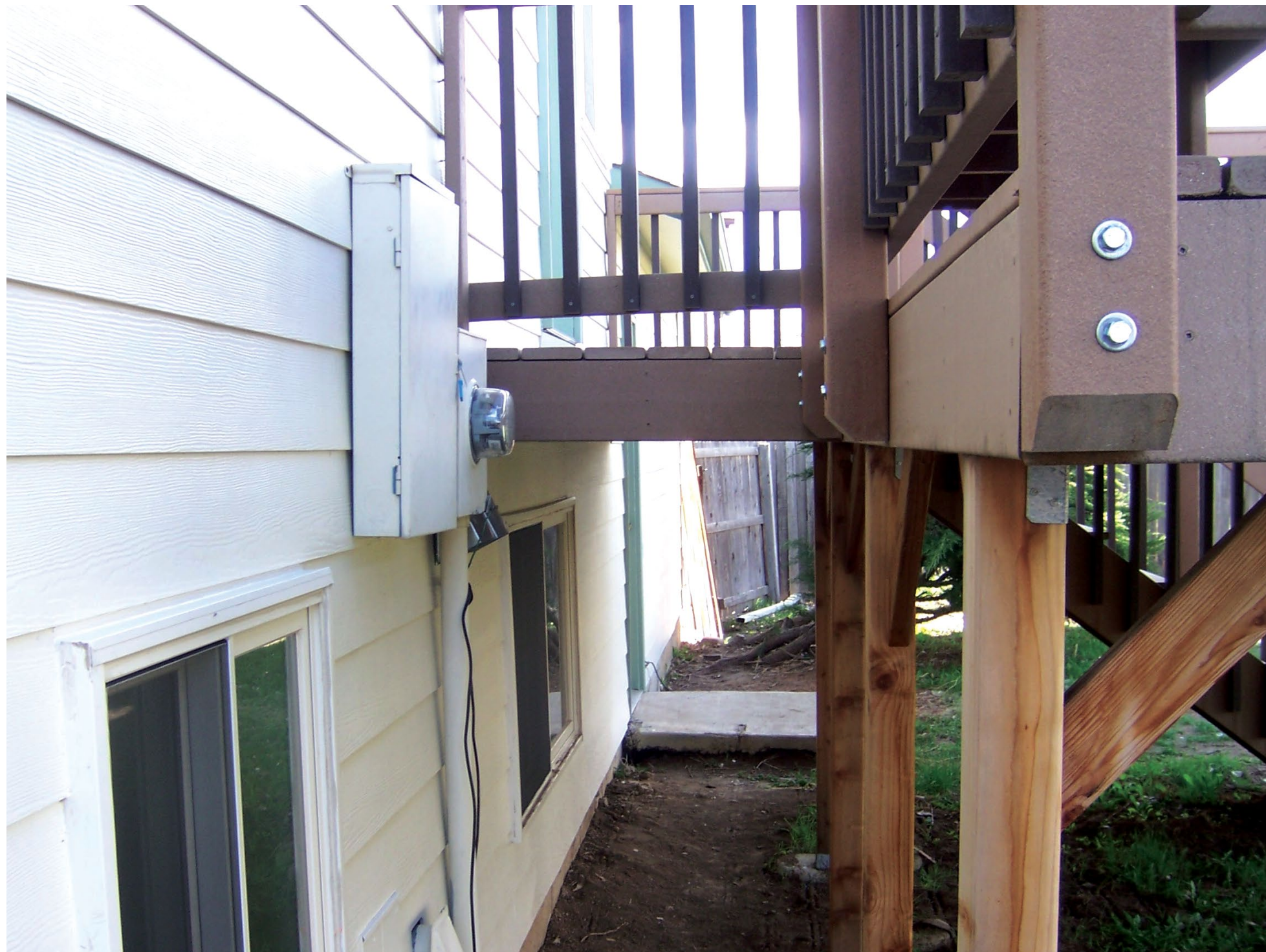
An example of electrical and emergency egress clearances.
