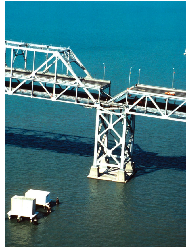
Loma Prieta, California, earthquake, Oct. 17, 1989. Roadbed collapse near the interface of the cantilever and truss sections of the San Francisco-Oakland Bay Bridge. View is northwest.
