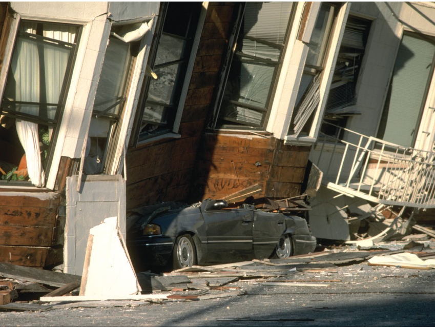
Loma Prieta, California, earthquake, Oct. 17, 1989, San Francisco. An automobile lies crushed under the third story of this apartment building in the Marina District. The ground levels are no longer visible because of structural failure and sinking due to liquefaction.
