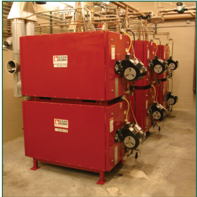
Figure 5 Oil-Burning Equipment Such as Listed Waste Class IIIB Oil Burners Used to Heat an Automobile Repair Facility are Exempt from an IFC Operational Permit. (Photograph courtesy of Clean Burn Energy Technologies, Leola, PA)
