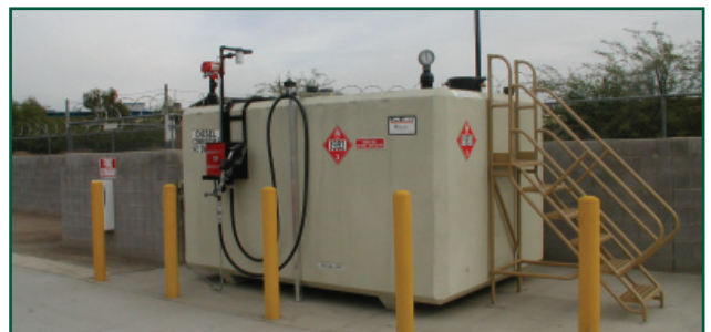
Figure 4 A 6,000 gallon, above-ground Storage Tank
