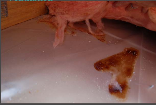
Case Study – Inadequate Ventilation
