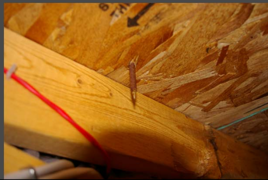
Case Study – Inadequate Ventilation
