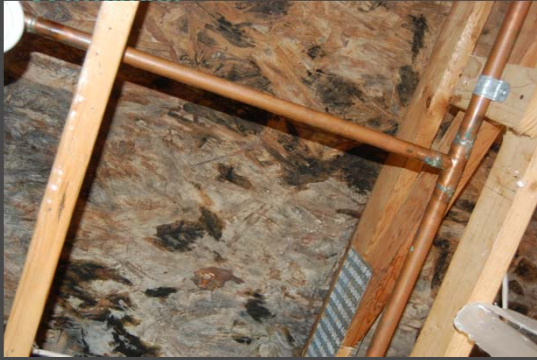
Case Study – Inadequate Ventilation
