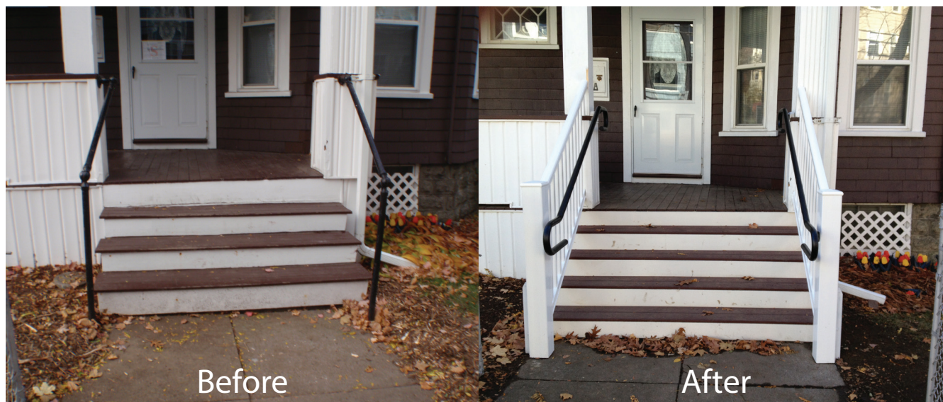
New front stairs with proper rise and run and new railings and handrails.
