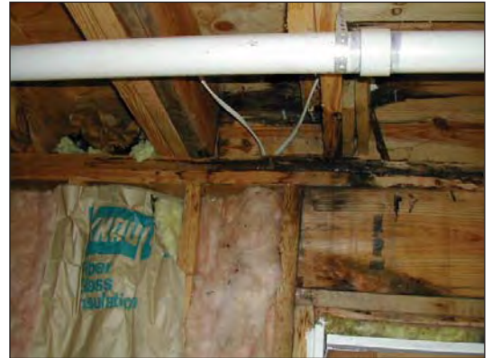
Severe water damage to the house framing can result from the lack of adequate flashing at the deck-ledger to house-band-joist connection.
