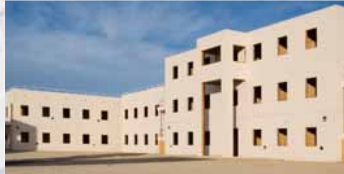
Construction crews install the Ecolite Metal Stud-Framed Lightweight Concrete Wall Panels at the U.S. Army's National Training Center in Fort Irwin, CA.
