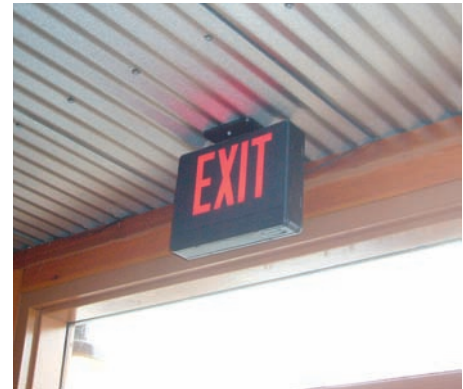
Internally illuminated exit sign.
