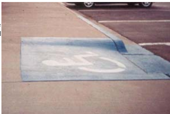
Figure 3: Curb cuts with side curbs and painted surface pose a possible tripping hazard.
