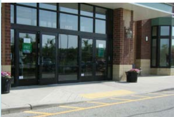
Figure 1: Example of a curb cut that has no top landing and is in a bad location for access to the entrance.
