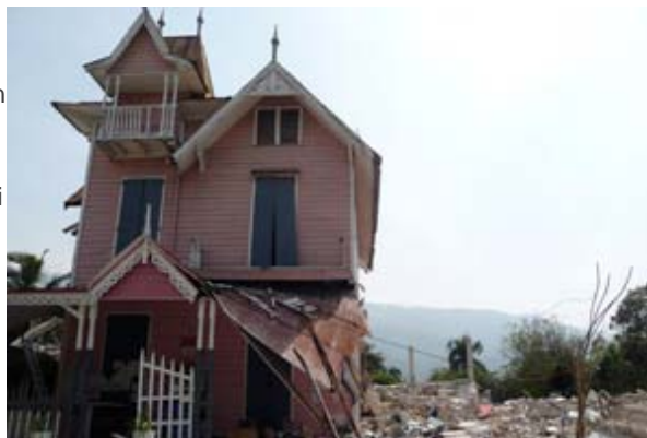
Wood frame building next to site of collapsed concrete building in Haiti. Photo by Martin Hammer.
