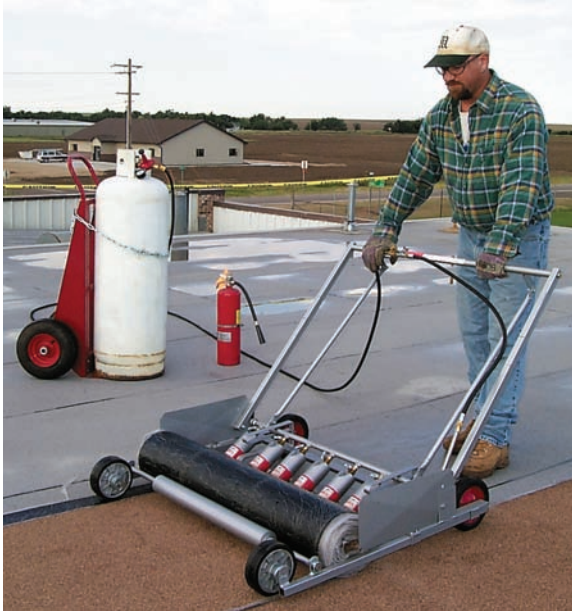
Portable cylinders on roofs are not prohibited by Section 6104.3.1. (Courtesy of Midwest Roofing Contractors Association, Glenview, IL)
