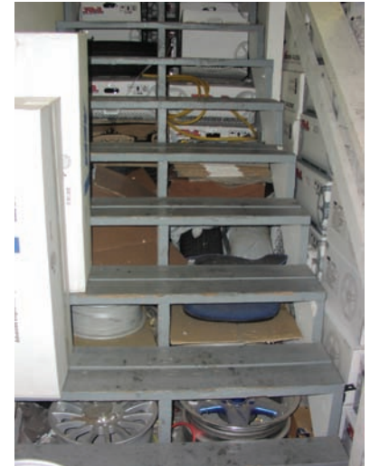
FIGURE 3-1 Storage of combustible materials beneath the egress stairs is a violation of the IFC. The concern is if the materials are ignited, this means of egress component is no longer available for the safe evacuation of the occupants
