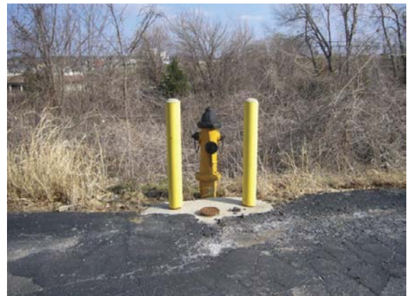
FIGURE 5-10 A fire hydrant with vehicle impact protection
