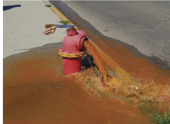
FIGURE 5-9 Flushing of a private fire hydrant to remove and discharge any sediment or debris in the private fire protection water main
