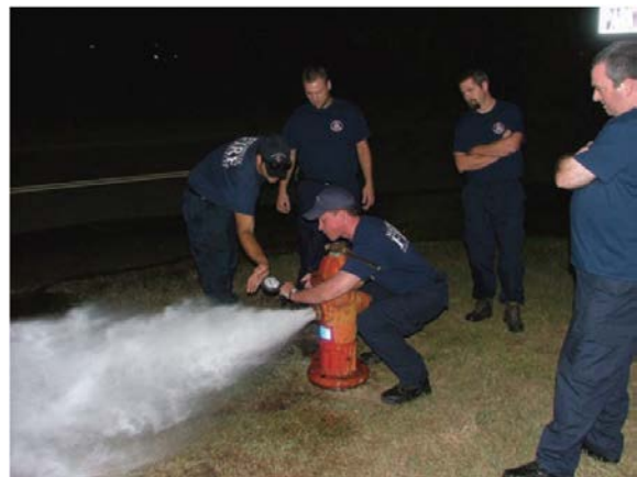
FIGURE 5-8 Flow testing of a fire hydrant to determine its available water supply
