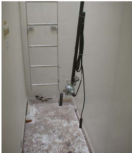
FIGURE 13-6 Devices such as these vapor and liquid leak detectors in a below-grade vaulted storage tank must be tested annually.
