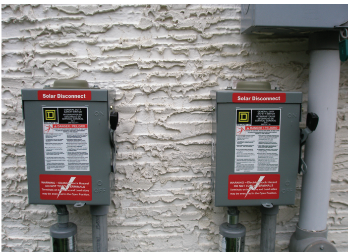
FIGURE 6-12 Solar photovoltaic disconnect switches
