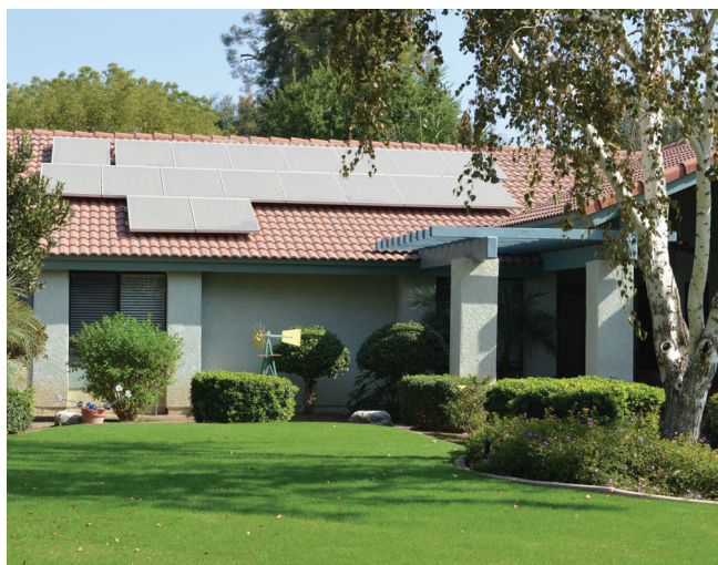
FIGURE 6-13 Solar panels on a one-family dwelling
