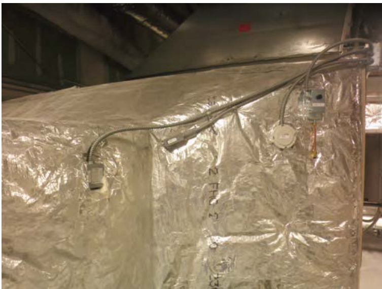
FIGURE 9-3 Monitoring devices are placed in this air-handling system, with efficiency data being transmitted back to a central computer monitoring station where the building engineer can make changes to the operation of the system if necessary
