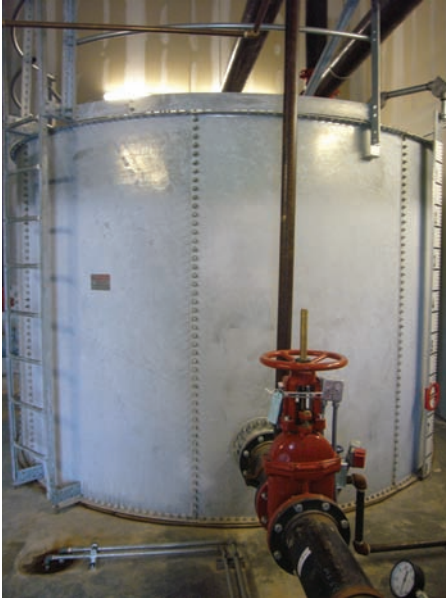
Tank providing secondary water supply
