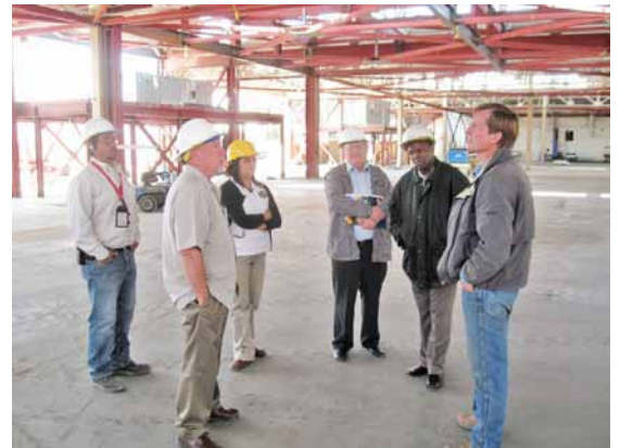
Oscar Davalos, Mark Gibbons, Preet Bassi, Kevin Bramwell, Joe Odhiambo, and Phil Delp at a seismic retrofit in Anaheim, California
