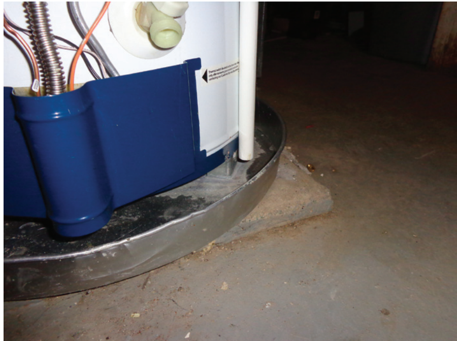
T&P discharge below flood level rim of pan
