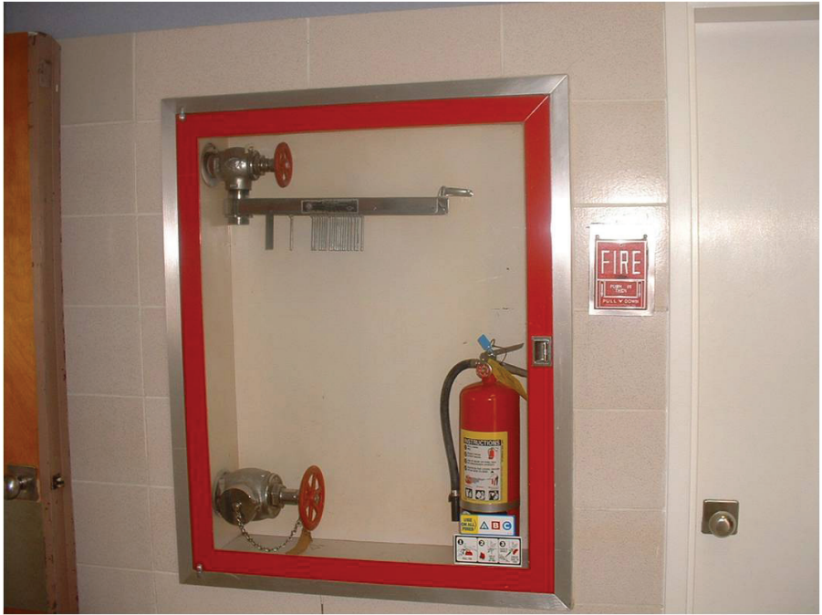
Hose and nozzle removed from an existing Class II standpipe hose cabinet
