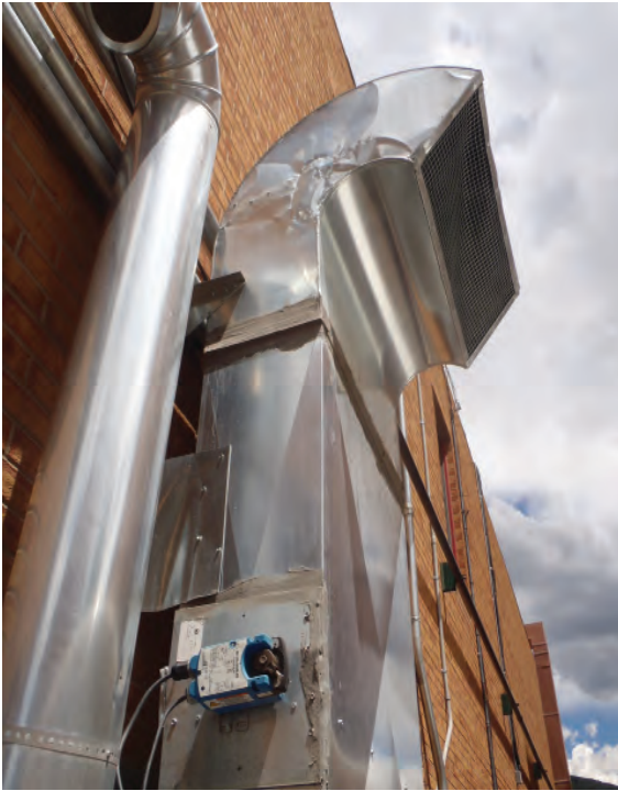
FIGURE 7-2 Motorized dampers control the air leakage through the air barrier.
