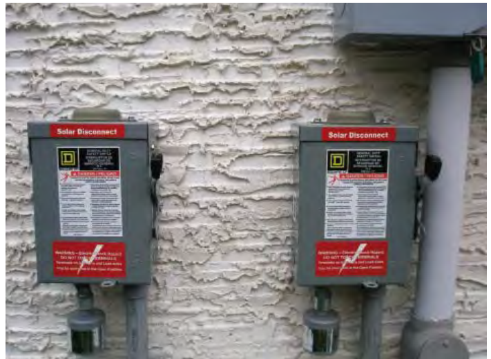
FIGURE 6-14 Solar photovoltaic disconnect switches
