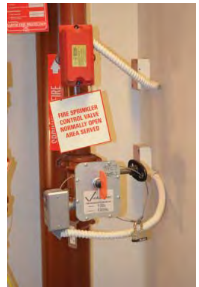
FIGURE 8-12 Electric supervision of an indicating floor control valve and water flow switch inside a high-rise building
