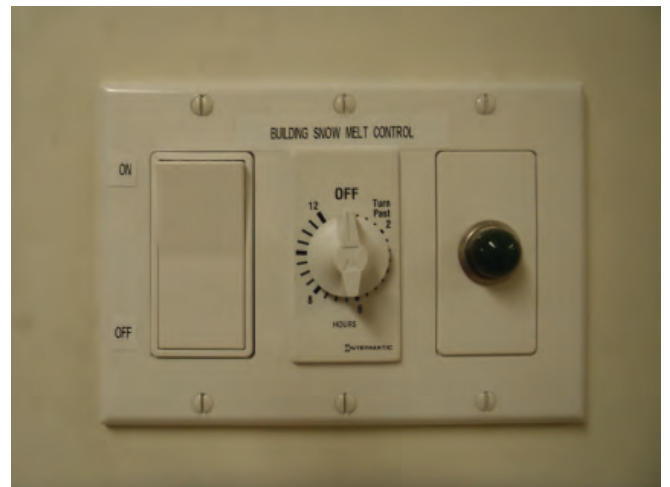
FIGURE 8-3 Manual control is allowed for complete shutdown.
