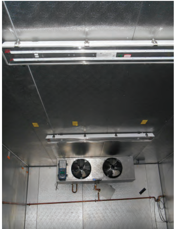
FIGURE 8-11 Walk-in cooler (Photo courtesy of A S Klein Engineering, PLLC)
