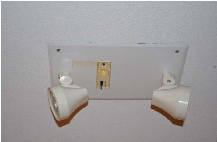
FIGURE 6-13 Emergency egress lighting unit with test button
