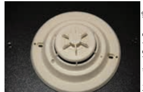
Smoke detector in R-2 occupancy
